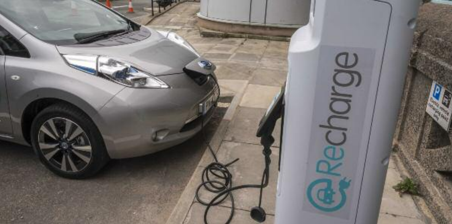
Vehicle Recharge point, Seacombe Ferry
